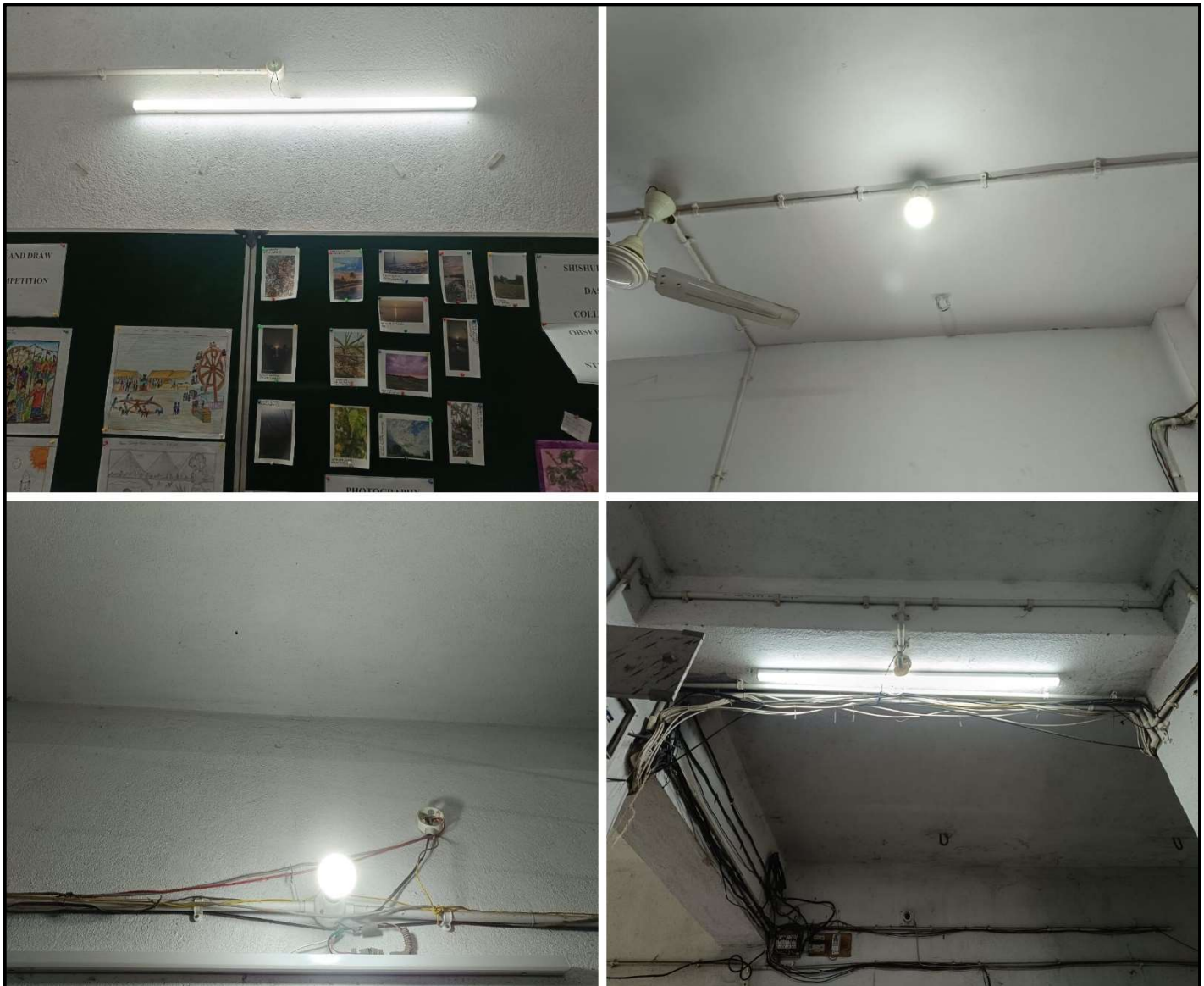
LED tubes and bulbs in use
